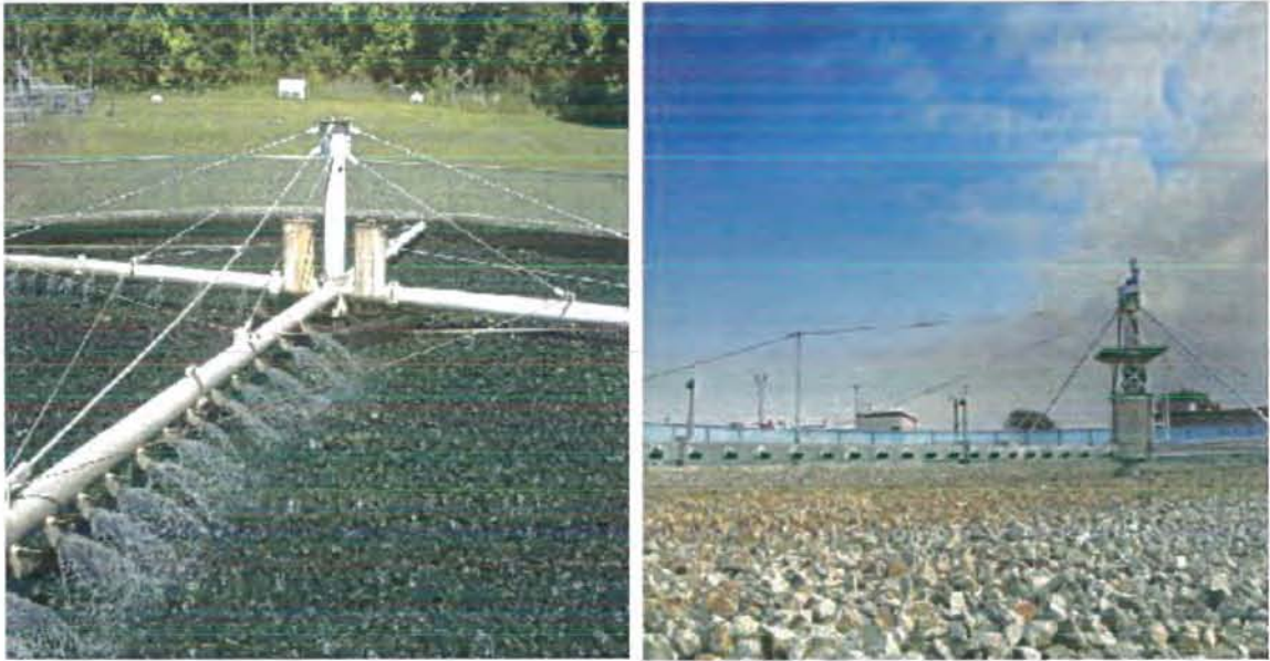
Fig. 2.3 Hydraulically driven rotary distributor (L); Electrically driven rotary distributor (R) (Adopted from https://www.environmental-expert.com/products/westech-biodoc-trickling-filter-rotary-distributor-2992 ).
