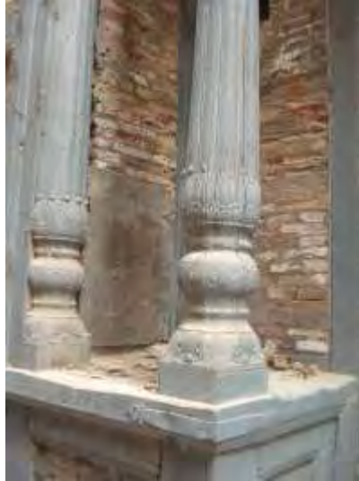
Fig.2.8 Pillars at the entrance of Raj Kapoor haveli . Photograph by researcher Dec2015
