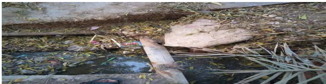
Figure 6: Damaged pipelines, mixture of drainage and sewerage lines.
