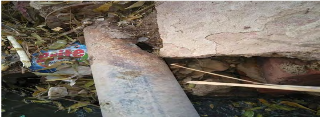
Figure 5: Damaged pipelines, mixture of drainage and sewerage lines.
