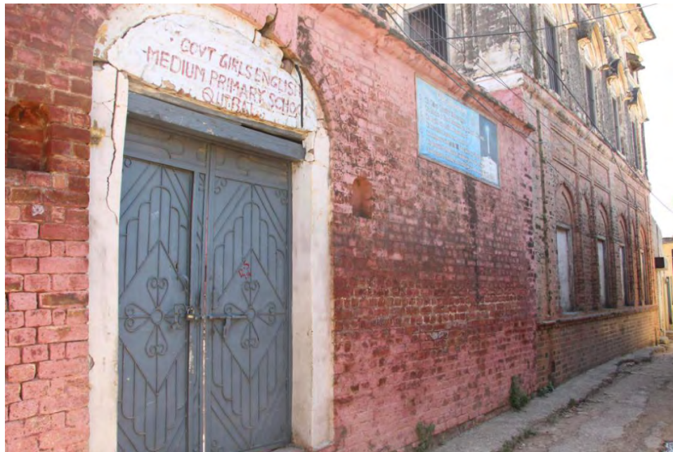
Plate 59 Outer wall and main entrance showing two rows of windows (Photo taken by Researcher)
