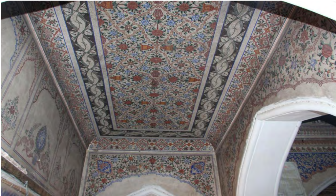
Plate 5.26 A rectangular roof panel thickly covered with floral designs and framed with two rows of border. (Photo taken by Researcher)
