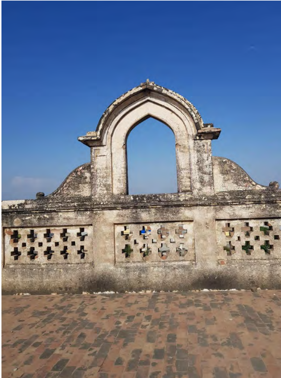
Plate 38 A small arch on fence wall at top roof (Photo taken by Researcher)
