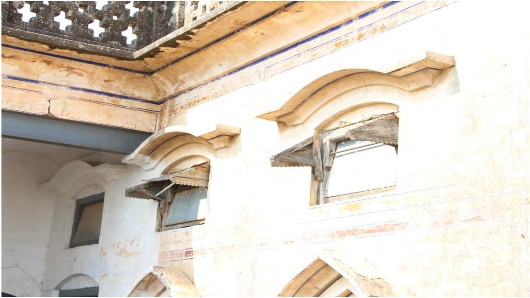
Plate 23 Shades over ventilators and windows used for decoration (Photo taken by Researcher)
