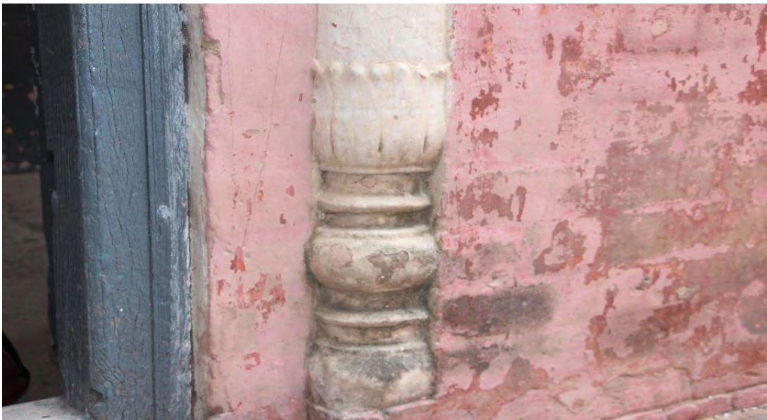
Plate 27 showing the base of pillar in outer wall (Photo taken by Researcher)
