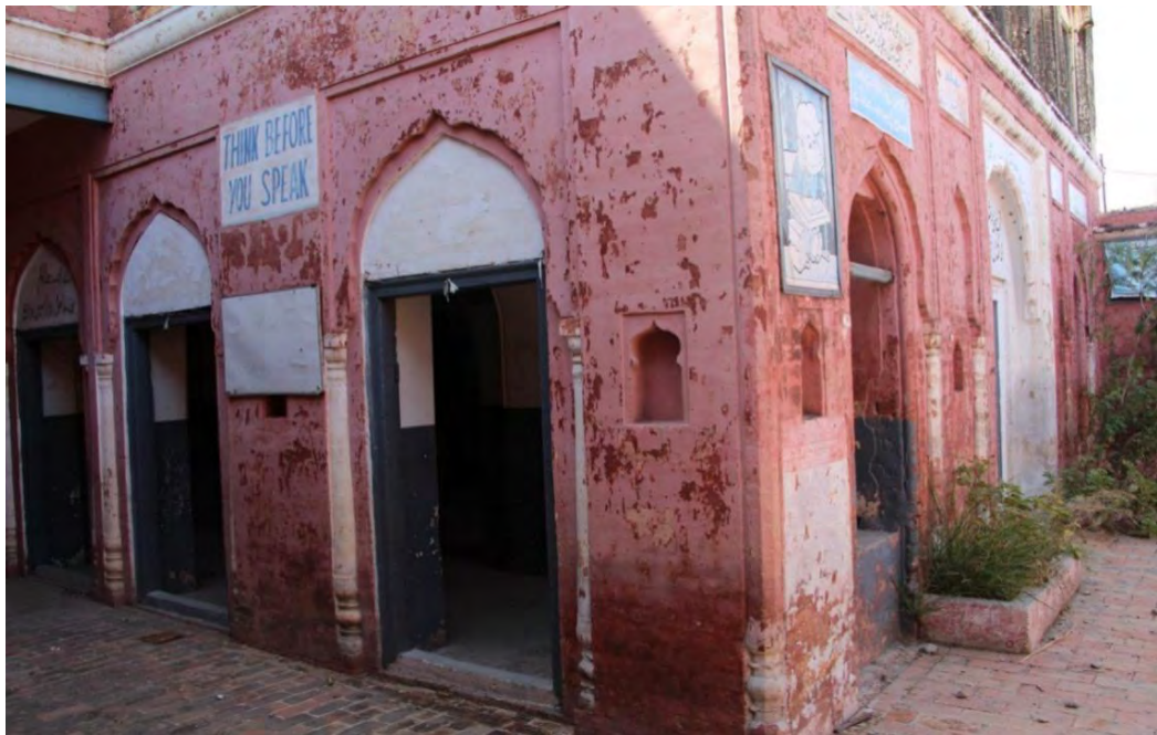
Plate 31 side view of Facade, southern wall with 3 arched openings (Photo taken by Researcher)
