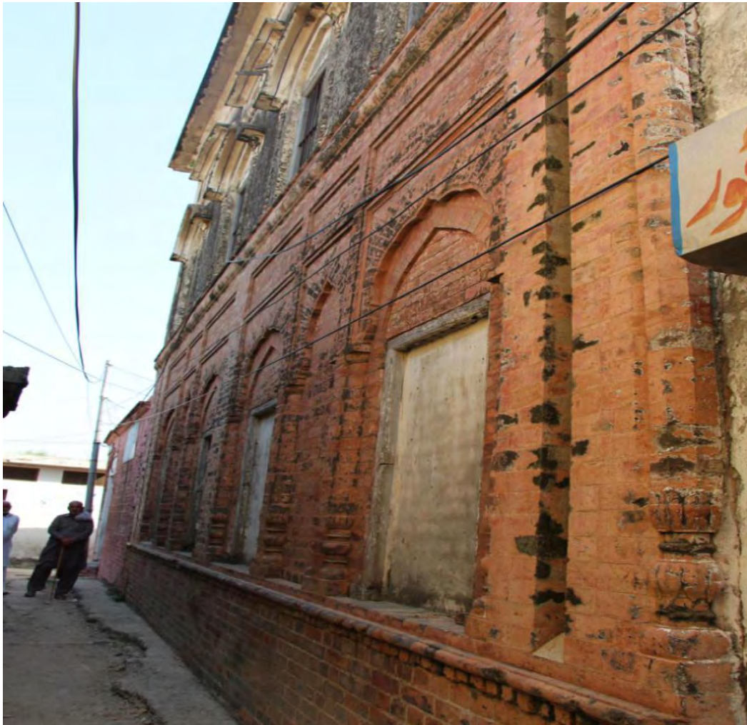
Plate 6 Outer wall of the building. Showing 4 arched windows now filled with bricks. (Photo taken by Researcher)
