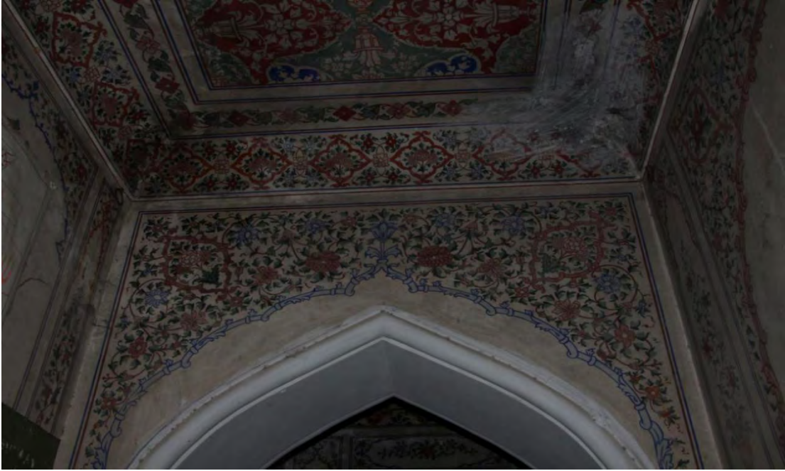
Plate 108 Art work done over arches in central hall. (Photo taken by Researcher)
