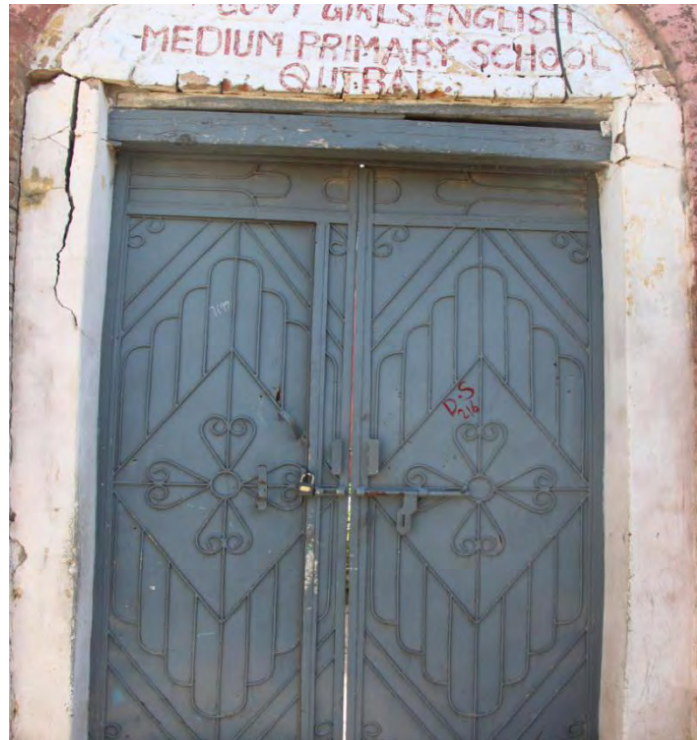
Plate 58 Entrance door now replaced with metal one (Photo taken by Researcher)
