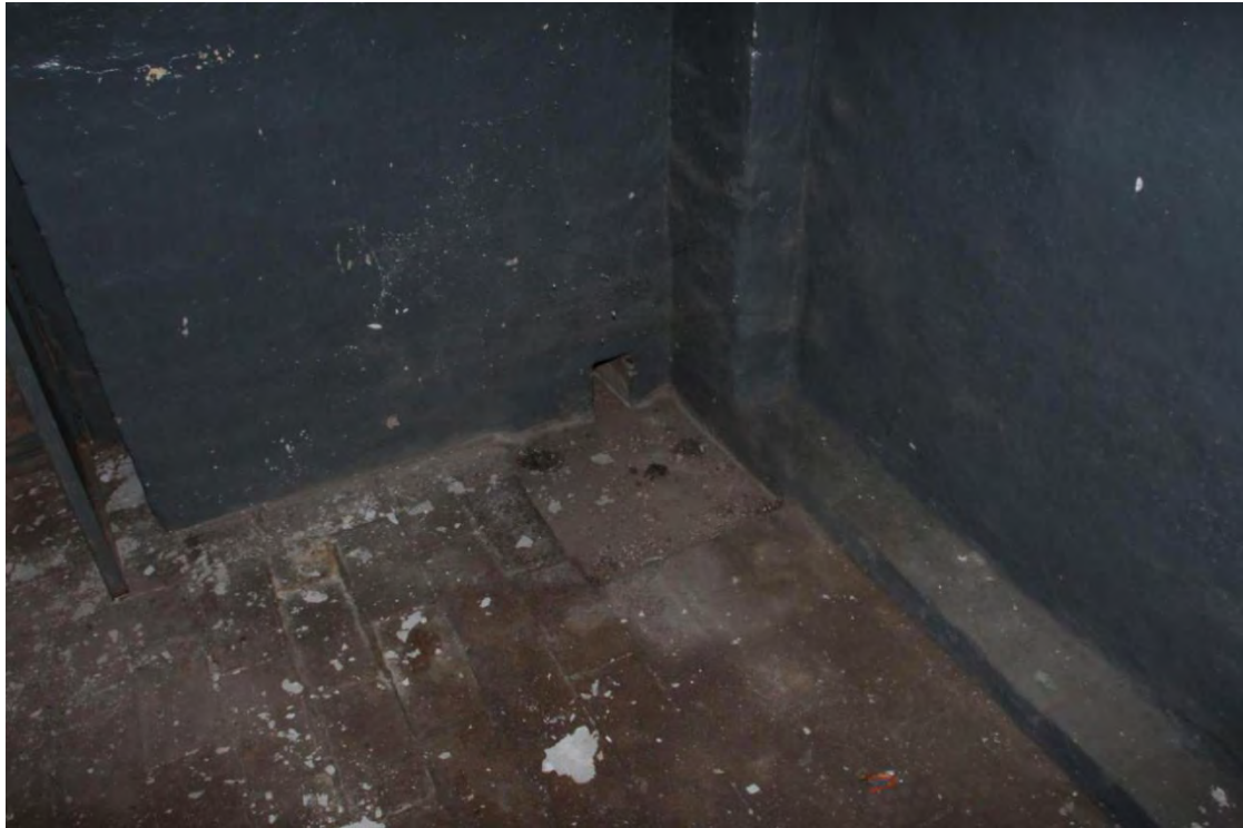
Plate 49 Drainage place at the corner of small rooms (Photo taken by Researcher)
