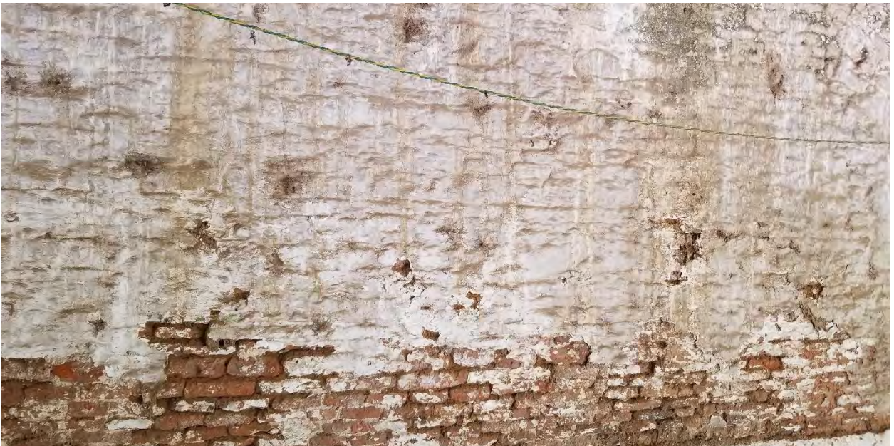
Plate 2 Remain of Southern Brick Wall (Photograph by Researcher)
