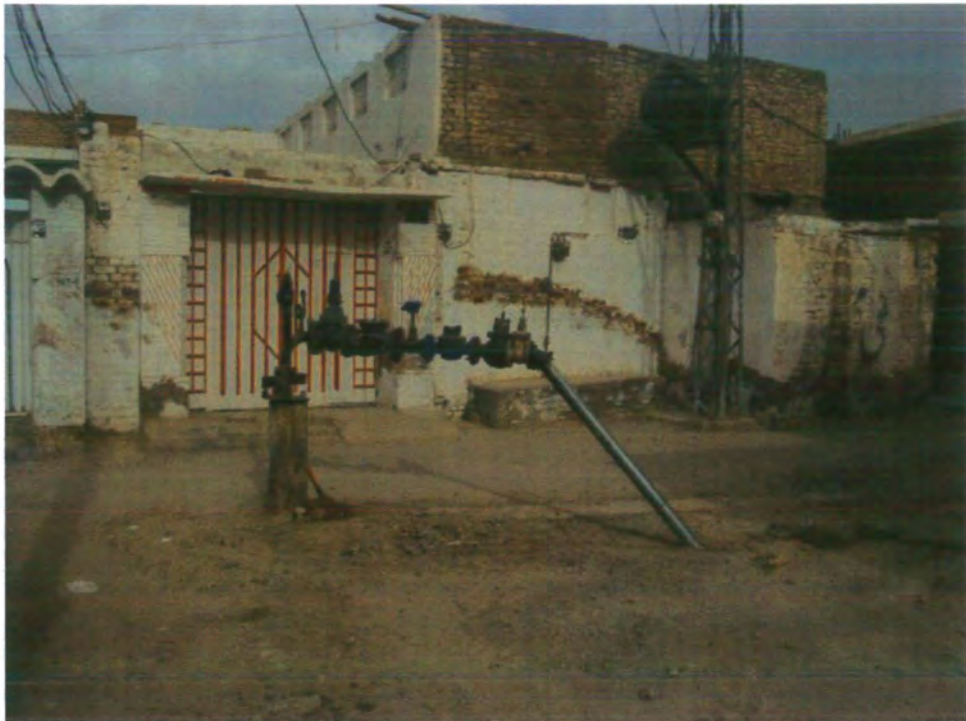
Plate 3: Water Pump of Bashir Abad Colony
