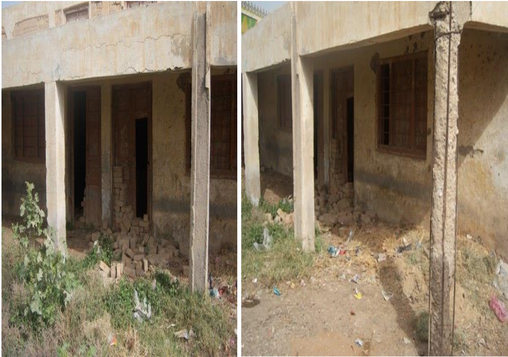
Figure 9: The structures show the story of affected schools
