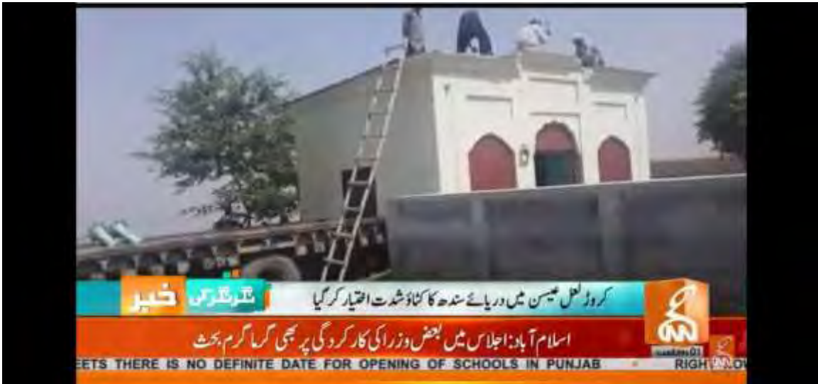
Figure 9. The community people are demolishing ( Shaheed ) mosque because of river bank erosion.
