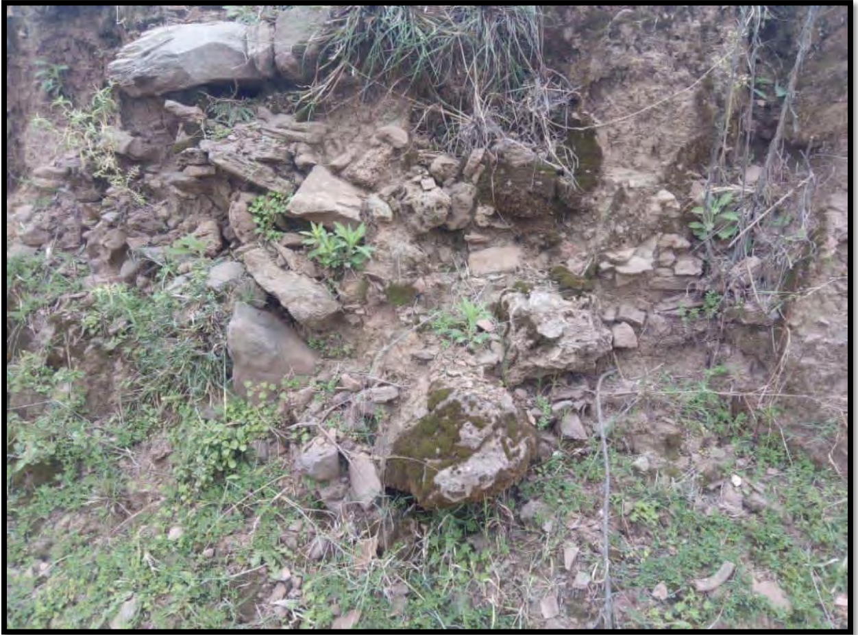
Figure 21: Wall Remains. (Picture taken by the researcher)
