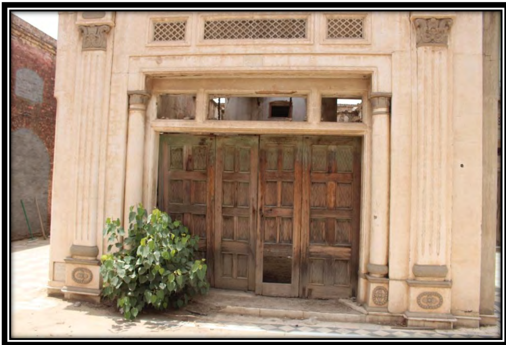
Figure 23: Main Entrance of the Sita Ram Mandir showing the Pair of Pseudo Corinthian fluted pilasters
