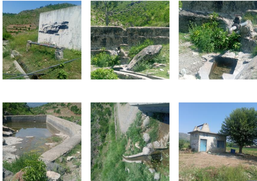
Figure 10 Nature's bounty harnessed: In Maloch, a robust concrete reservoir stands tall, capturing rain and spring water, powering an advanced irrigation system that cultivates prosperity across the village
