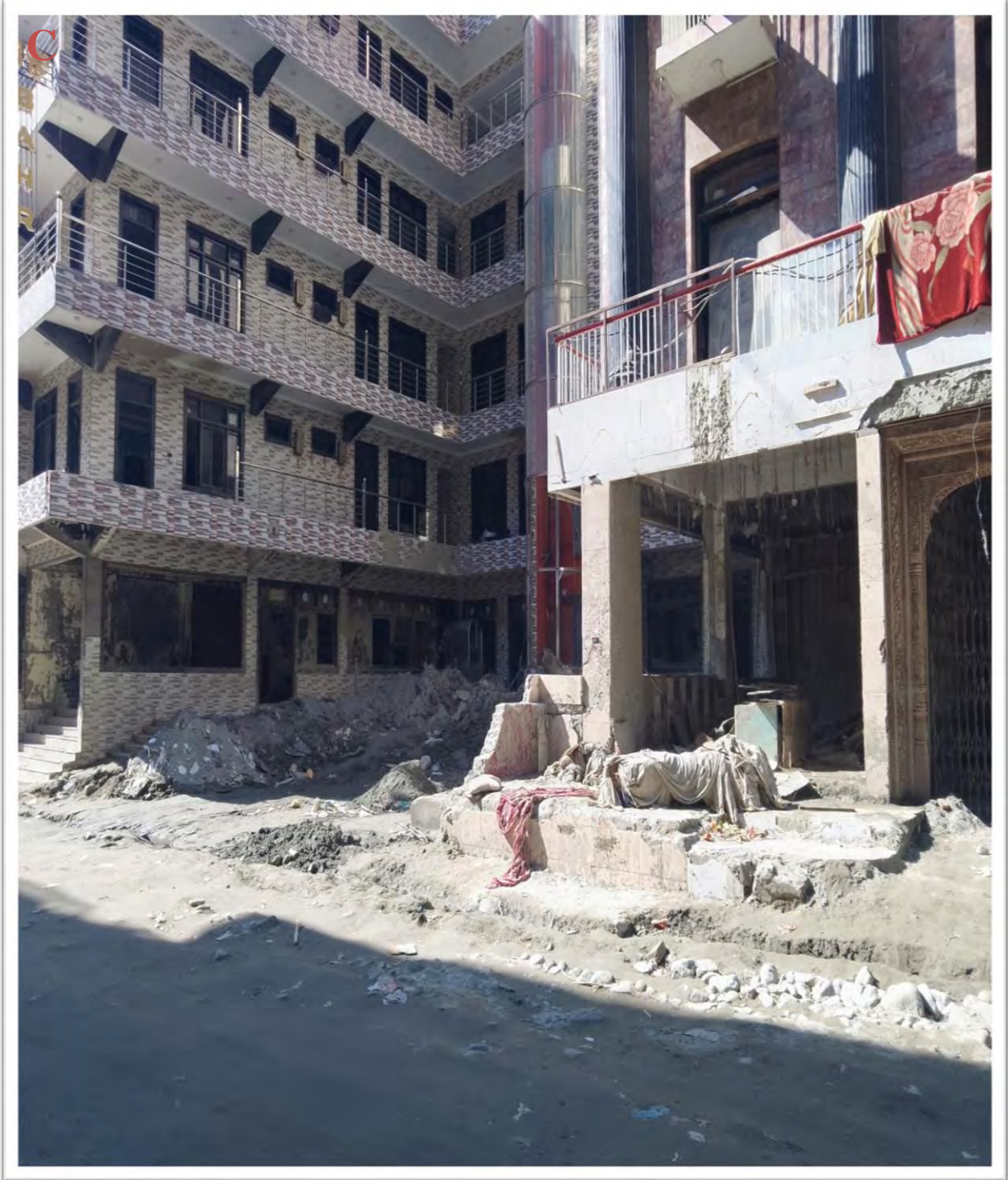
Figure 3.3 C The buildings are completely destroyed and cracked during 2022 flash flood. Figure showing the buildings which are the most expensive first class hotels of the main Bahrain city.
