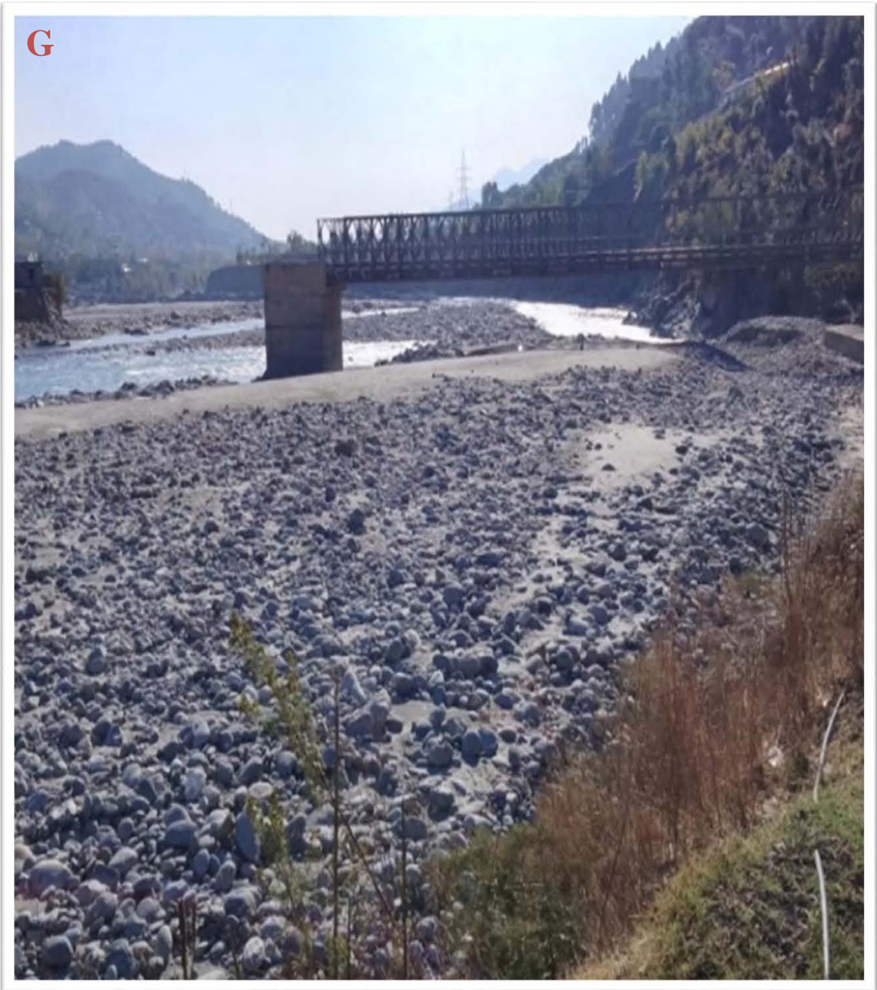
Figure 3.5 G Impacts of debris floods on overpass of Qandeel Gari. They were completely destroyed in flash flood as shown in figure
