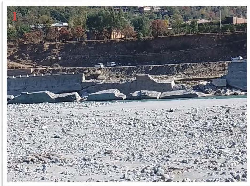
Figure 3.3 H and I Qandeel section the infrastructures and main highway slides to the river. The river banks are destroyed Terraces are also damaged and fractured as indicated in figures.
